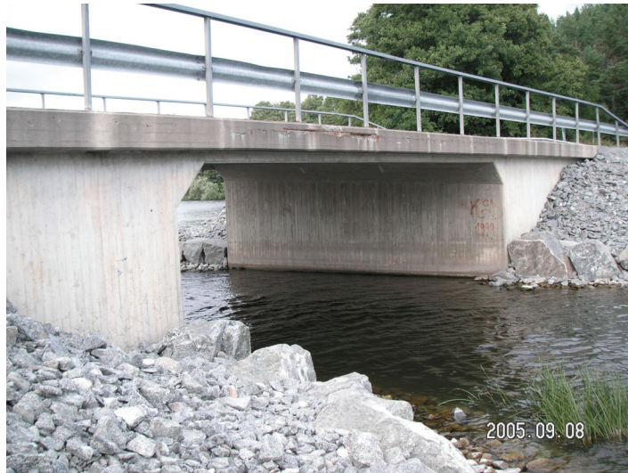
Figure 4.5. Bridge C72 in Uppsala County. This slab frame bridge (concrete) was built 1982 and has a bridge area of 92 m 2 .
