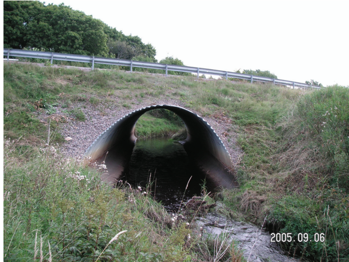
Figure 4.11. Bridge C143 in Uppsala County. This culvert (steel) was built 1966 and has a bridge area of 101 m 2 .
