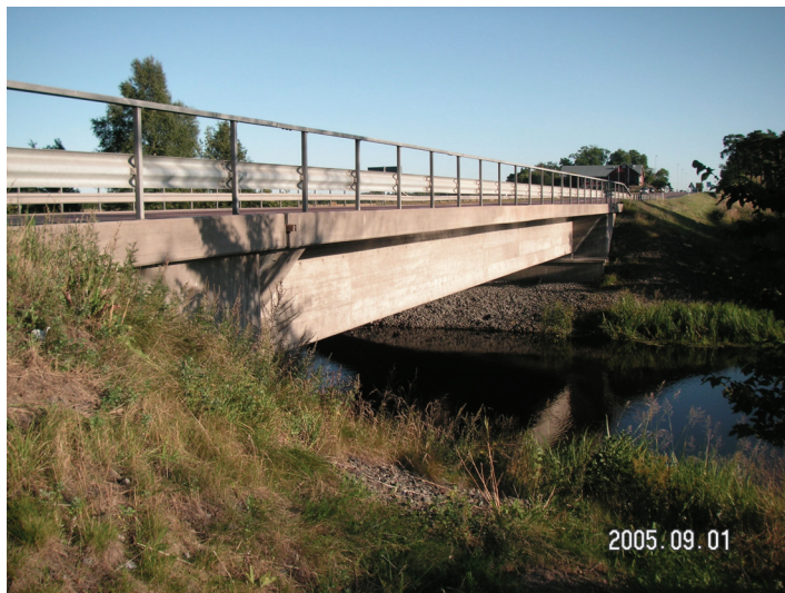
Figure 4.3. Bridge C56 in Uppsala County. This beam and slab bridge (concrete) was built 1985 and has a bridge area of 440 m 2 .
