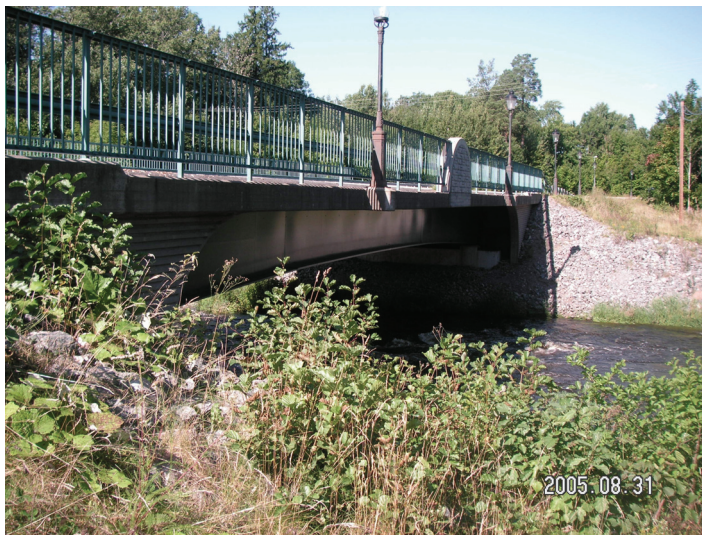
Figure 4.9. Bridge C616 in Uppsala County. This beam and slab bridge (steel) was built 1995 and has a bridge area of 418 m 2 .
